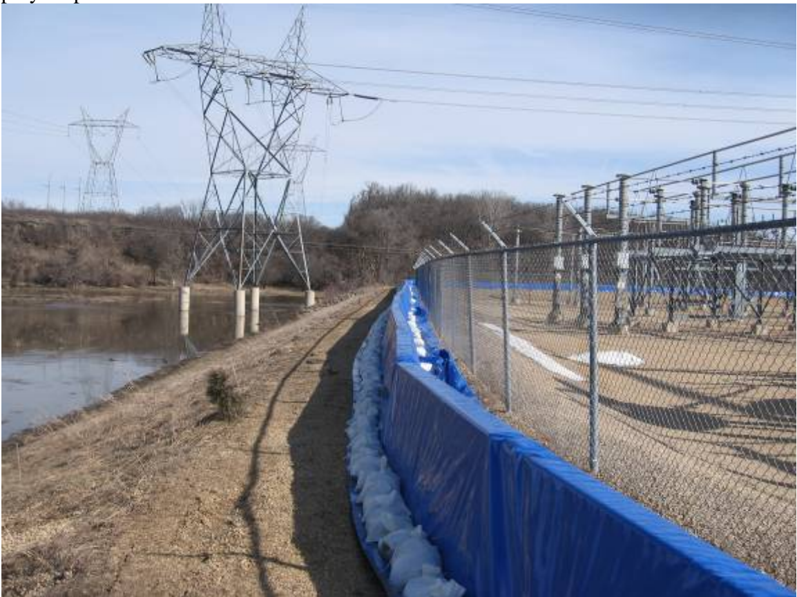
Completed flood wall. A pump was also staged onsite to handle any infiltration or rain events.
