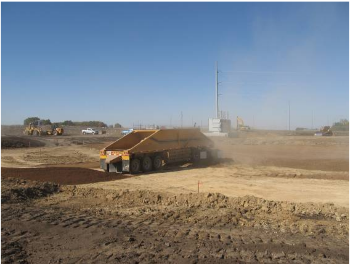
Grading and soil corrections to enlarge and upgrade an existing substation in Western Minnesota
