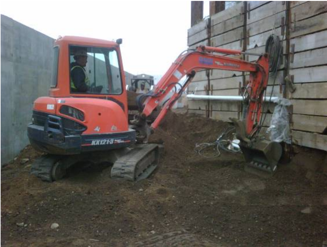
Working around a soldier pile and lagging wall used to protect existing building foundation during rock removal and tank construction.
