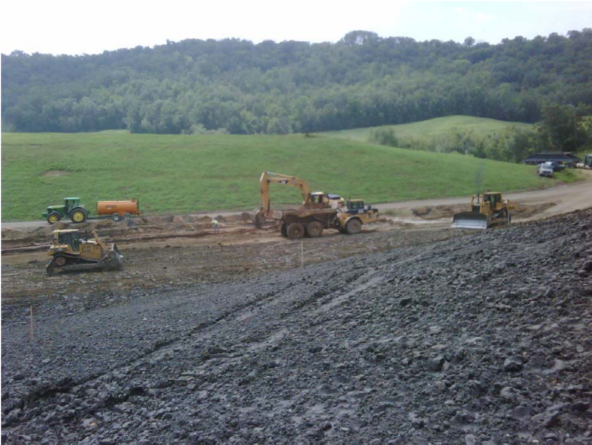
Sub grade finishing and clay liner placement for a new cell at an ash containment landfill in Minnesota.
