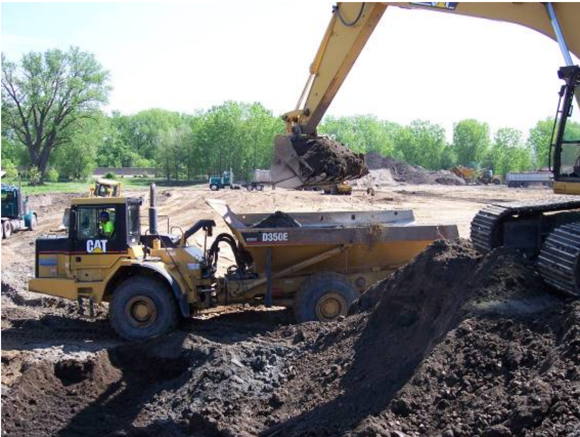
Grading for SSP Cleanup project. Job consisted of onsite earthwork, processing excavated soils, exporting contaminated material, and importing clean material to grade site.
