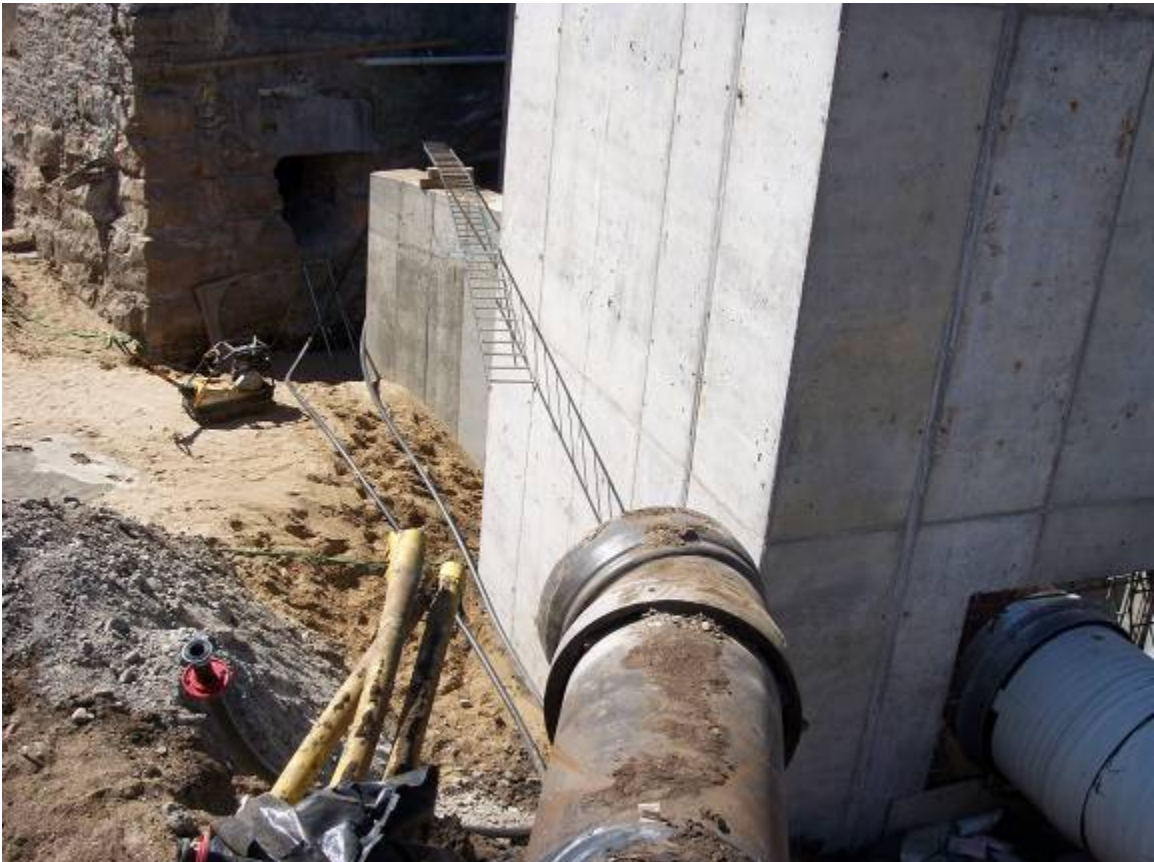
New lines tied into existing lines at the Minneapolis Pump House Project
