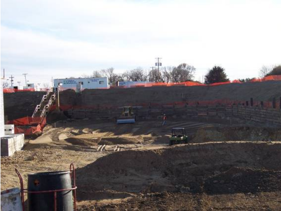
Backfilling and fine grading for new Digester next to soldier pile and lagging wall used for temporary support of flood levee.
