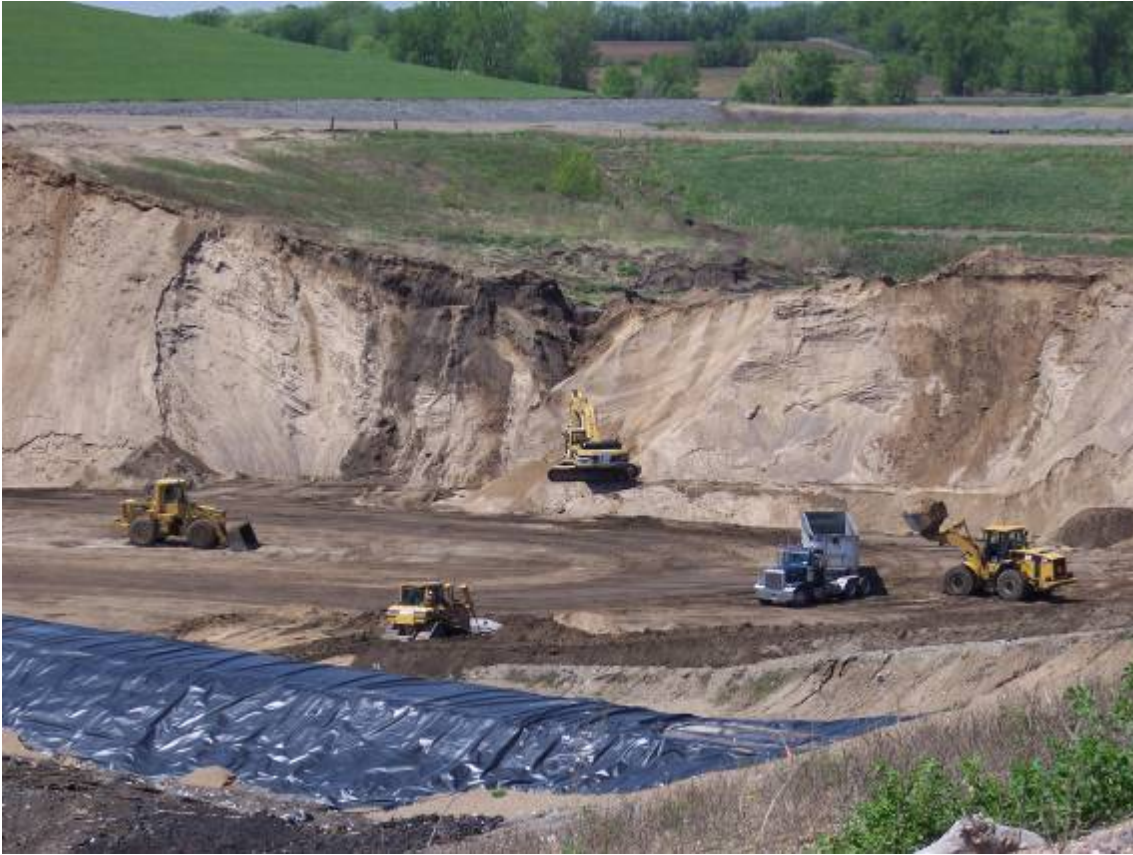
Excavating and grading at Landfill as part of our South St. Paul Cleanup Project
