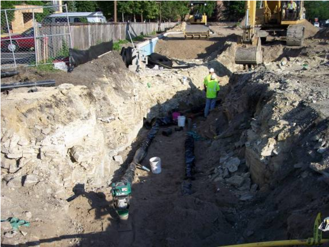
New water services for a new assisted living facility in St. Paul, MN. We had to rip and hammer rock for all the utilities on this project site.
