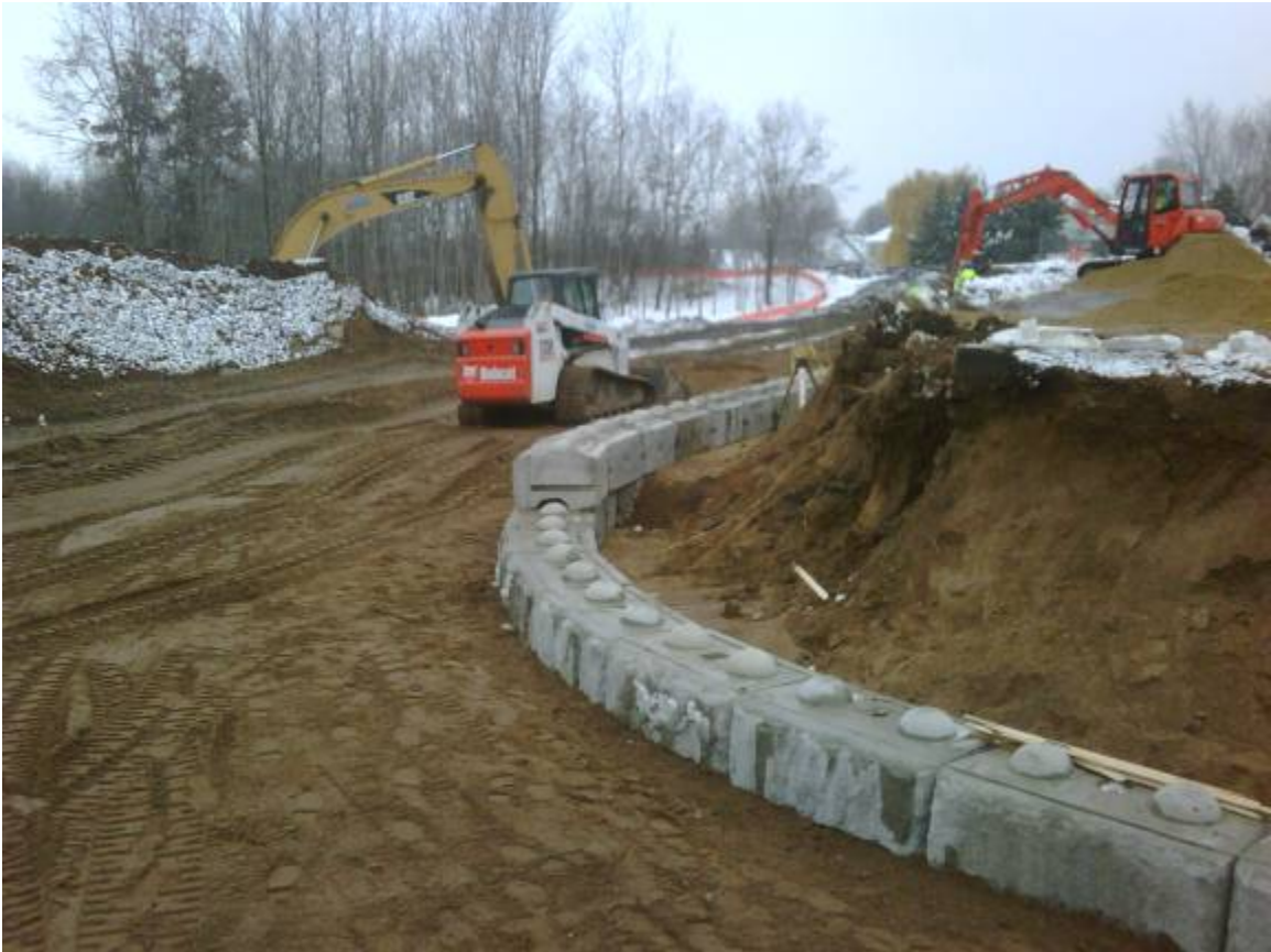
Retaining wall constructed by Dahn Construction in Burnsville. The wall was suggested to the owner as an alternate to the soldier pile and lagging wall in the bid documents. This VEP saved the owner money, schedule time, and provided a more scenic landscape.
